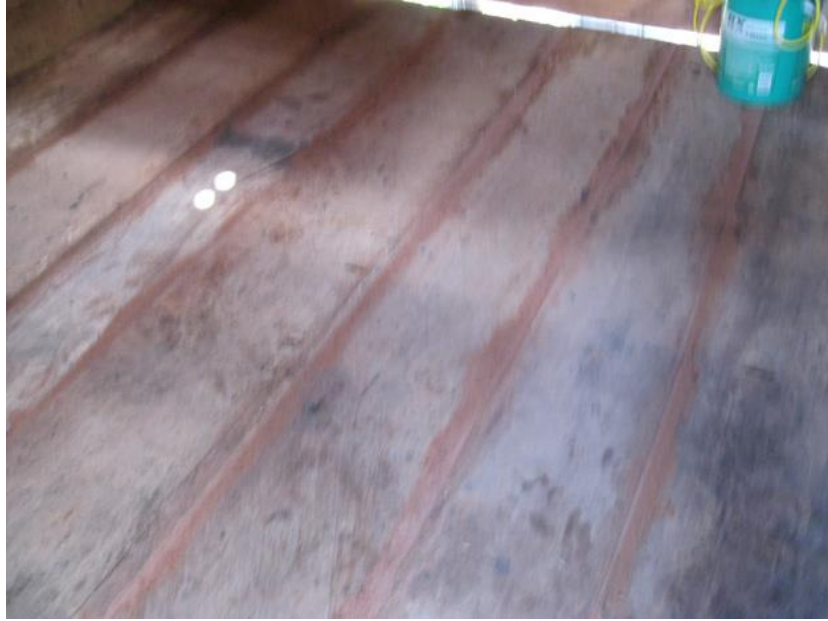
Sealed floor board in house.
