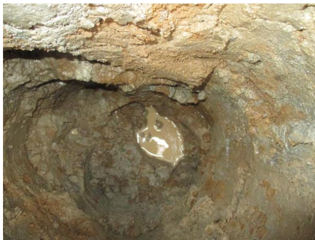
Water entering test hole in seep.
