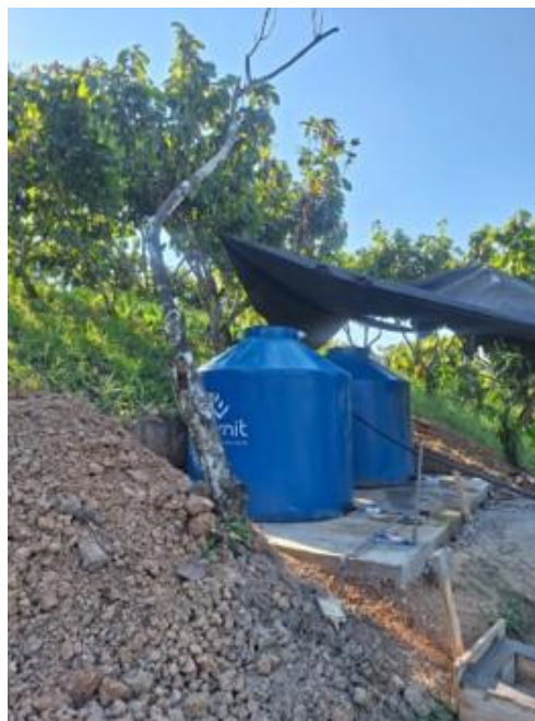
New water tank location and support pad.
