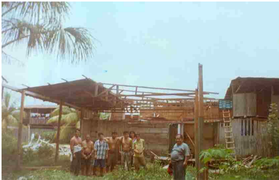
Construction of the church in Palcazu (Pablo Paredes extreme left, Manuel Villar on the far right)
