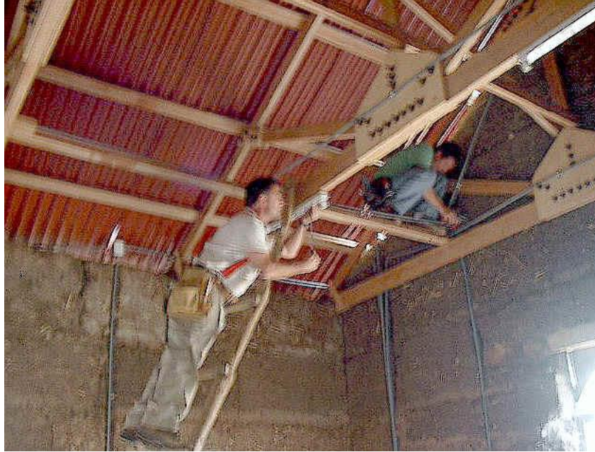
Scott and Rob, members of the Sugar Hill team installing the electrical system in Ahuac.
