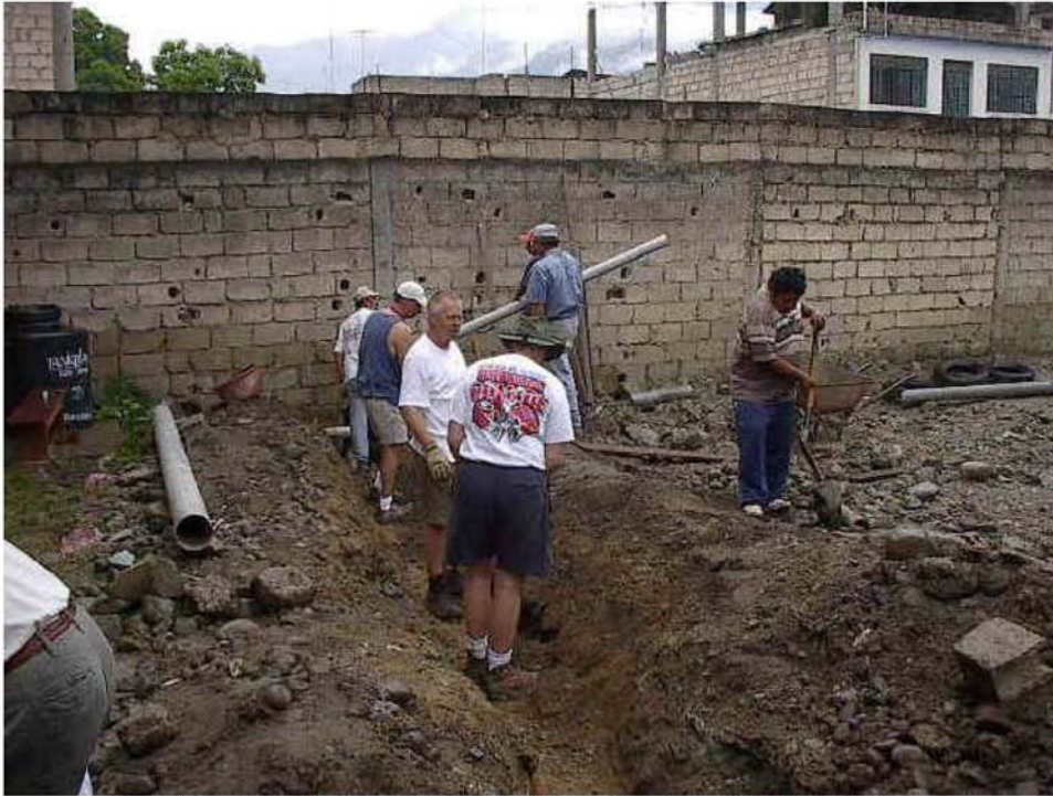
Team from Alpharetta First United Methodist Church installing sewer line at San Ramon
